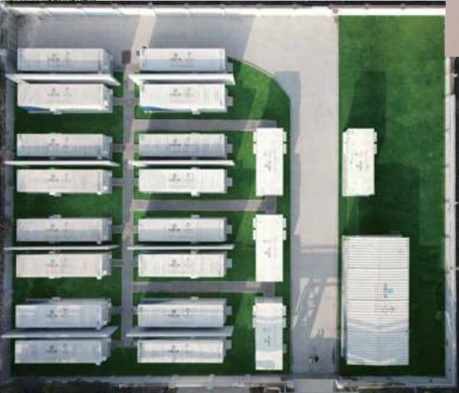
10MW/39MWh Energy Storage Station
